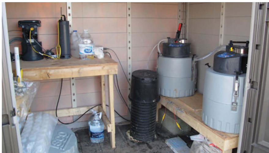
Instrumentation used to monitor tile water flow and sampling collections on one of the farm field sites.
